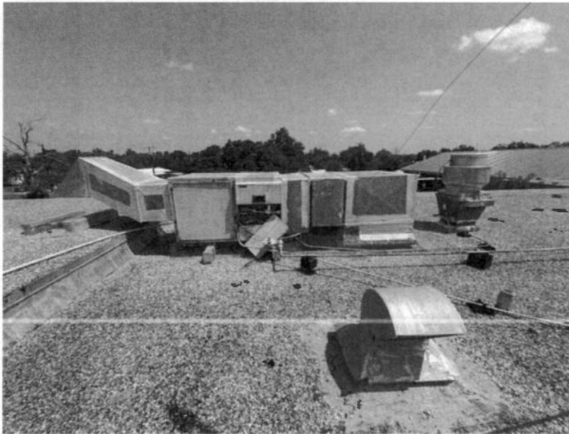
Abandoned RTU to be removed.
