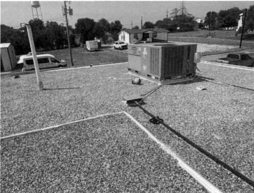
RTU will have to be lifted to access the underlying curb.
