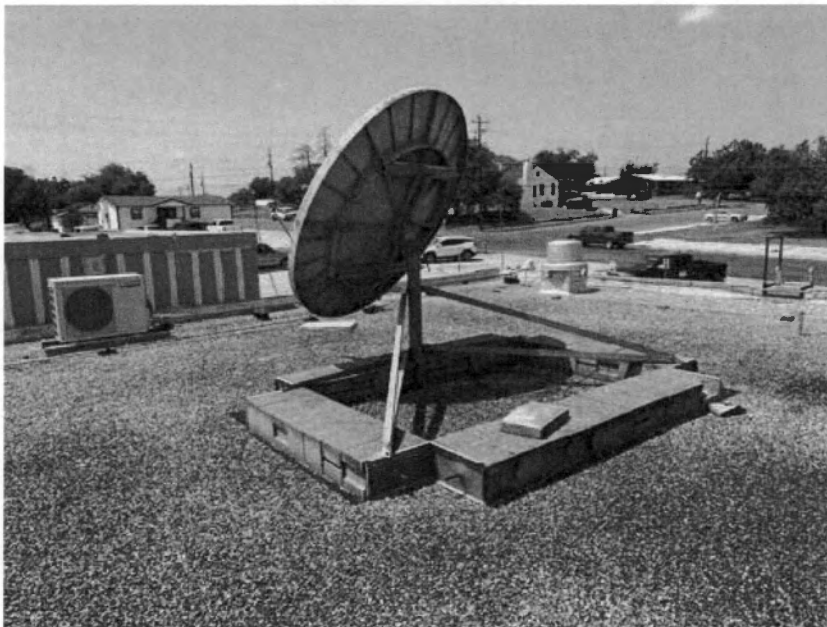
Satellite dish to be removed as it is non-functional.
